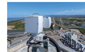
BU-43U outdoor remote camera installed on a building rooftop
